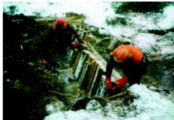
Constructing a wooden dam in a ditch in Olvassuo Strict Nature Reserve
