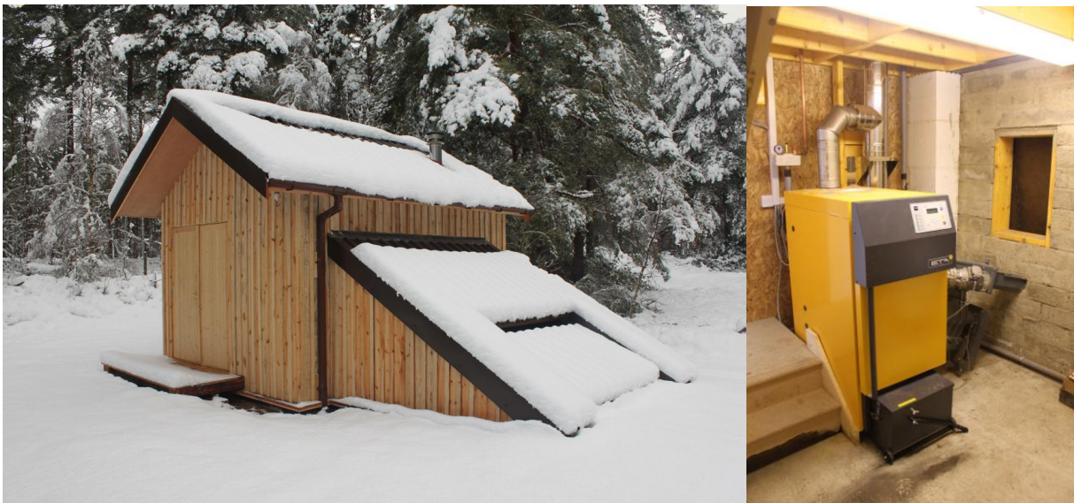
Highland Birchwoods woodfuel boiler and shed
