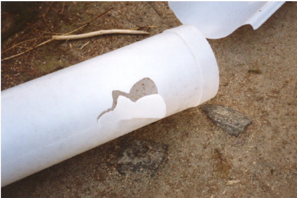
Plate 6 Damaged Section at the Road
